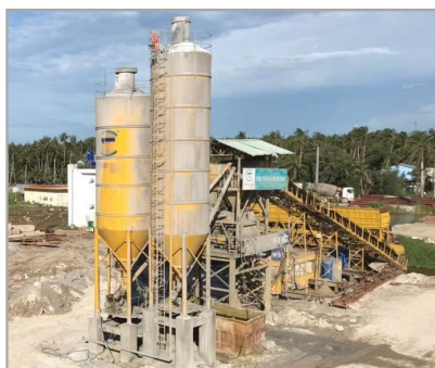
TRẠM TRỘN BÊ TÔNG 90M 3 CONCRETE MIXING STATION 90M 3
